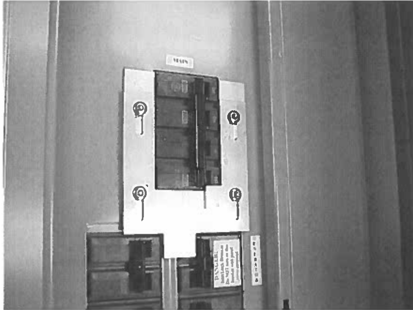
Photograph A-9 K-8010 INTERLOCK KIT (As Installed)
